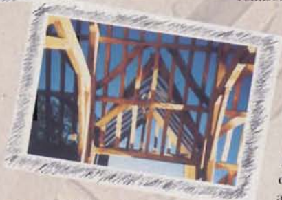
In progress: the massive, skeletal oak frame. Following the storms of 1987, the Burlinghams bought a quantity of oak at a reduced price. They stored it at a sawmill and visited it once a year when buying the family Christmas tree.
