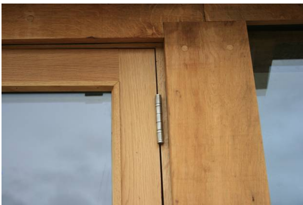
Fig 1: The unit to the left of the main post is a glazed door, typical of a joinery item with a frame which sits within the primary structure. On the right of the main post is a surface mounted fixed pane, where no secondary frame is required and therefore the whole aperture is glazed.
