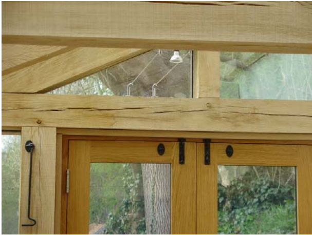
Fig 6: Detail of joinery frame mounted to the main frame on the external posts. Beadings are attached internally to cover the gap which will appear between the frames as the green elements shrink.
