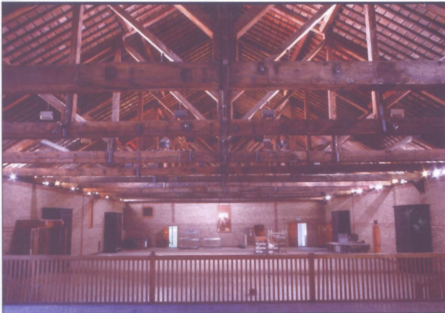
Figure 2.16 Concealed stainless steel rods strengthen these trusses at the Porter Tun Room
